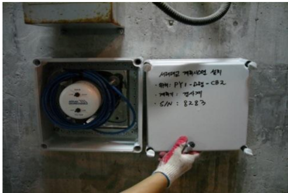
Figure1. Installed tilt-meter at pier
