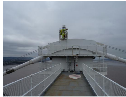
Figure 4. The GNSS antennas located at survey point T2 on the bridge. The illustration shows the GNSS antenna being installed.
