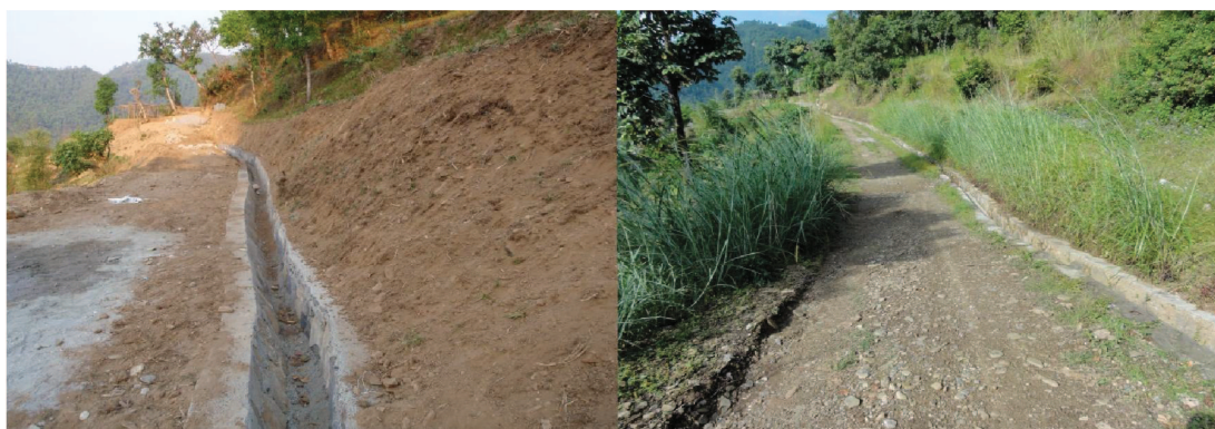
Figure 6. Left: Gharelu village, Kaski District after drainage structure and slope modification in April, 2014. Credit: K. Sudmeier-Rieux; Right: same site in November, 2014. Credit: G. Leibundgut.
