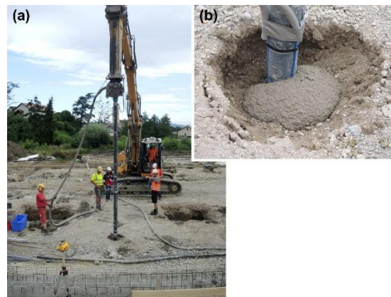
Fig. 2 (a) Pile during construction and (b) detail of a pile with \varnothing 118 mm with surrounding material
