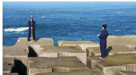
Figure 11 – Coordinating a GCP. The greenish colour of the surface of the blocks is due to slime
