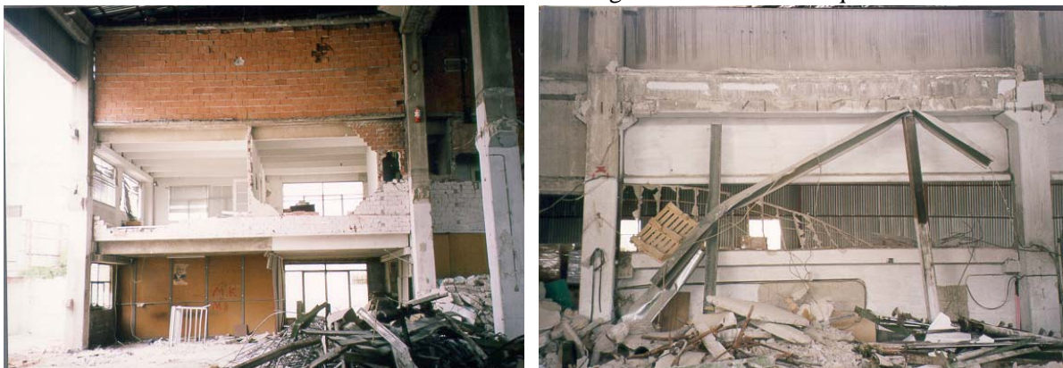
Fot.1: Internal condition of the building after the 1999 earthquake
