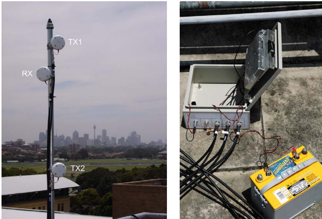
Figure 2 Example LocataLite (5) antenna setup and weatherproof enclosure.
