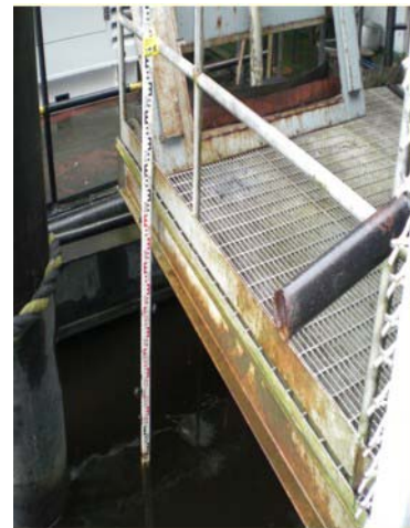
Tide Gauge Installation at the project area.
