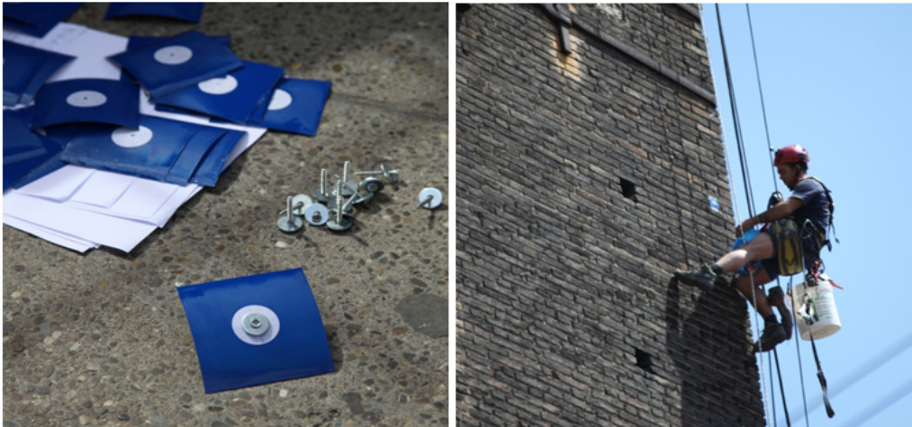
Figure 2: Reflective targets used for the registration (on the left); targets installation on the tower's wall (on the right). In each tower at least eight targets were placed in every wall, close to the edges and equally distributed along the tower's extent.
