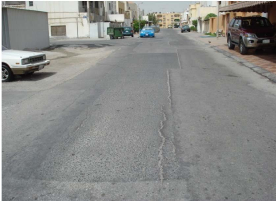
Figure (1) Roads Defect need maintenance (Cracks on the asphalt)
