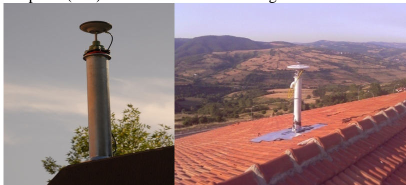
Figure 4. Galvanized steel pillar (4 m from the base of roof)
