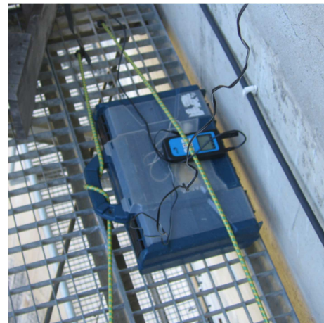
Figure 17 – Digital thermo-hydro-barometer on the walkway
