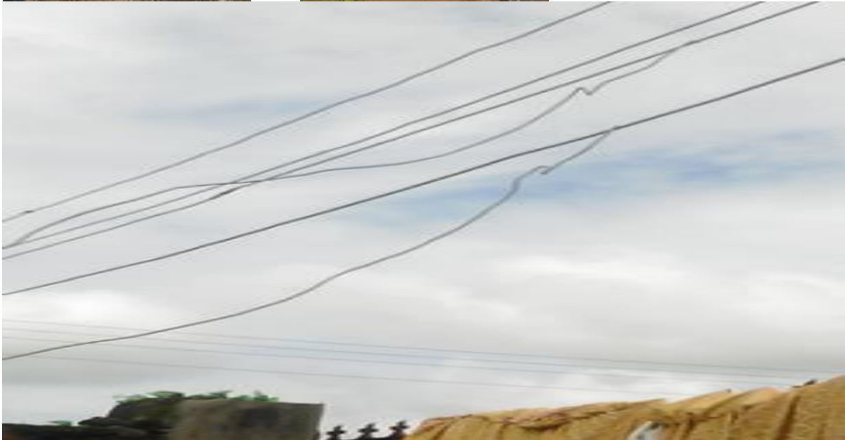
The level of pot hole and damage surface and illegal connection of electricity in World Bank Housing Estate
